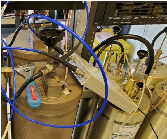
(The TR1300/1 is shown, connected to the receive leg of a DB4060 duplexer. Both return loss and rejection loss were adjusted on this duplexer.)
